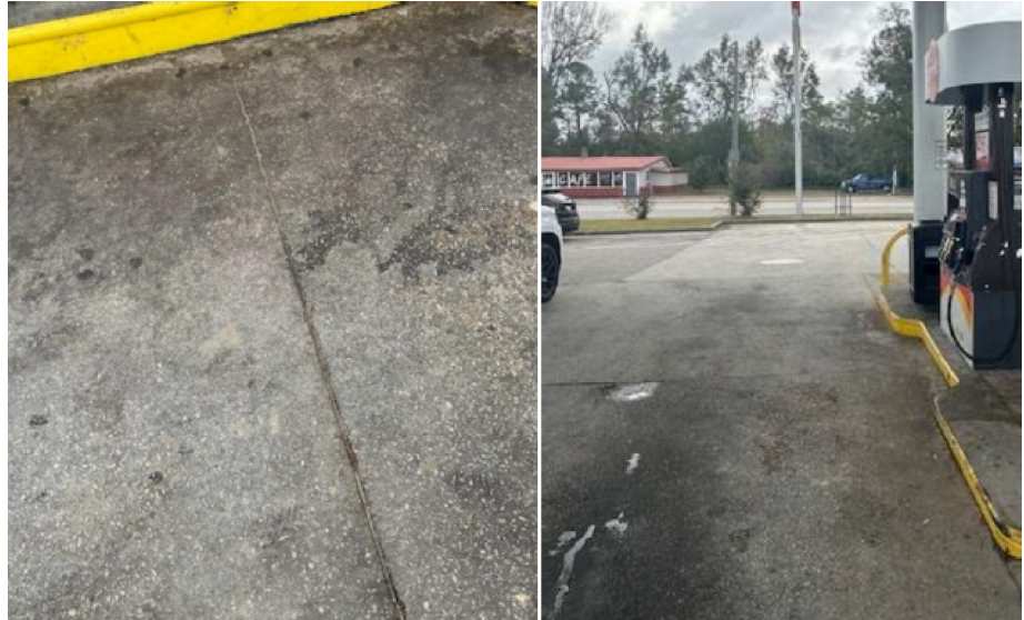
The area of the parking lot near the pumps where Walker fell
